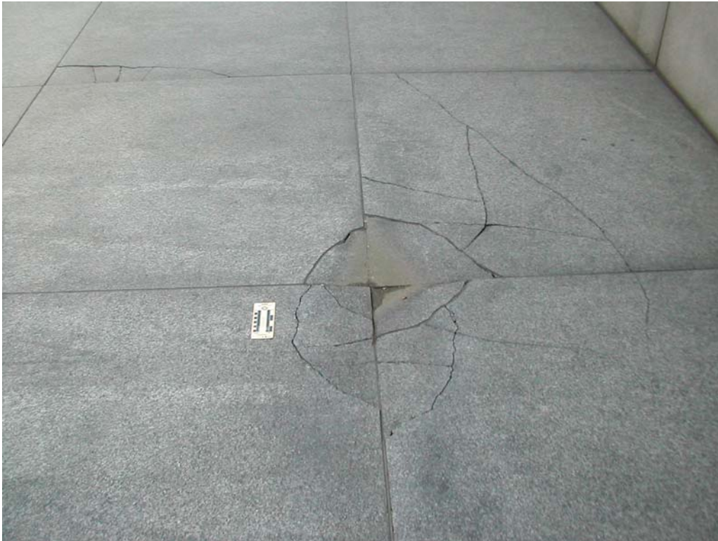
Figure 2: Deformation of the expensive granite pavers due to subsidence of the fill materials (plastic scale is 1 foot).
